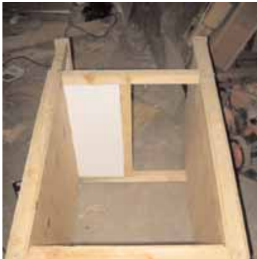
Only half of the front wall is open. The other half is insulated with polystyrene.
