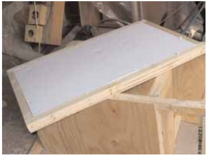
...filled with foam. Plywood sheathing covers both sides. I recommend covering the floor with linoleum.
