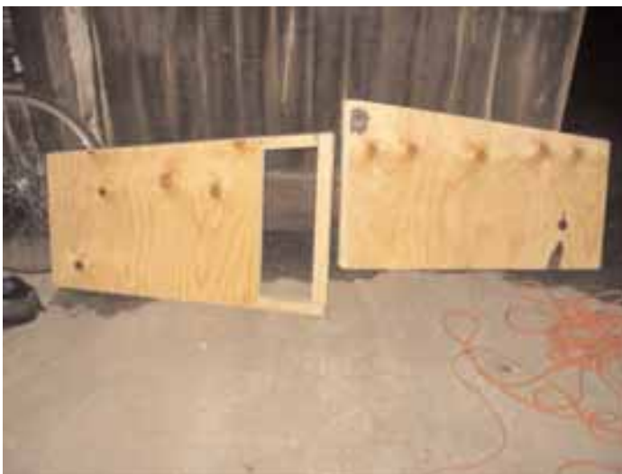
Left and right walls with sheathing in place. Nowhere is the polystyrene exposed to the cats. See door?
